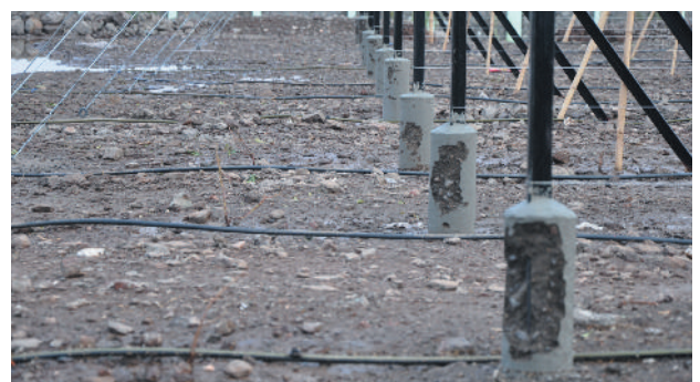
Damage to cement base of grapevine trellis
