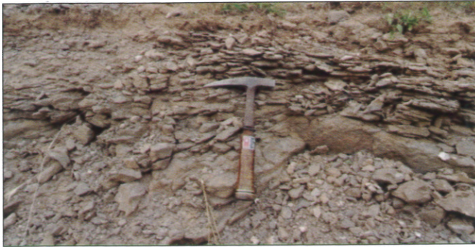
Fig.45. Weathering of upper horizon of vesicular flow where rocks have been weathered along the fractures and cracks
